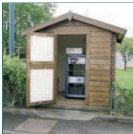
Station de surveillance de Saint-Jean-de-Braye.
